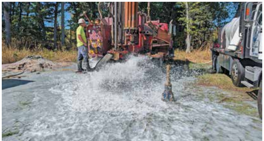
Drilling the rock (air purge through the drill string brings cuttings and water up from below)
