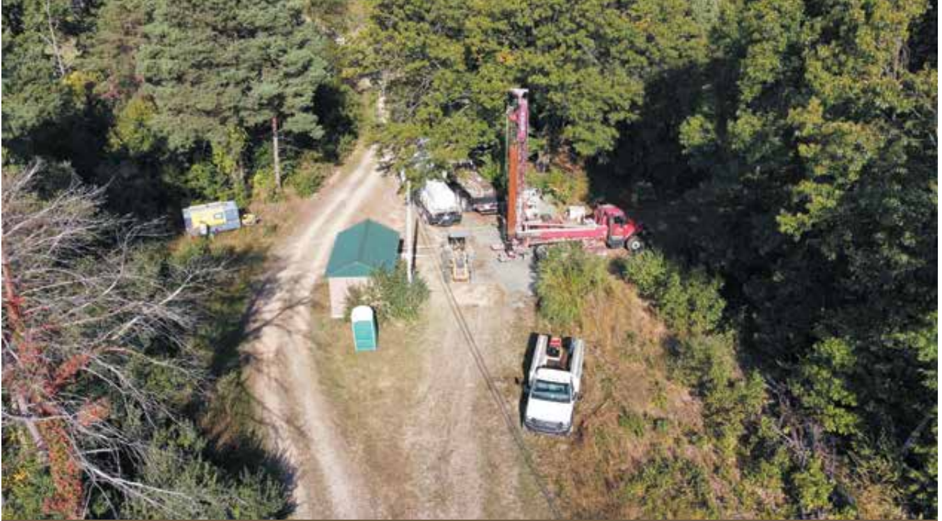
One of 22 new well sites (note the proximity to the existing well house)
